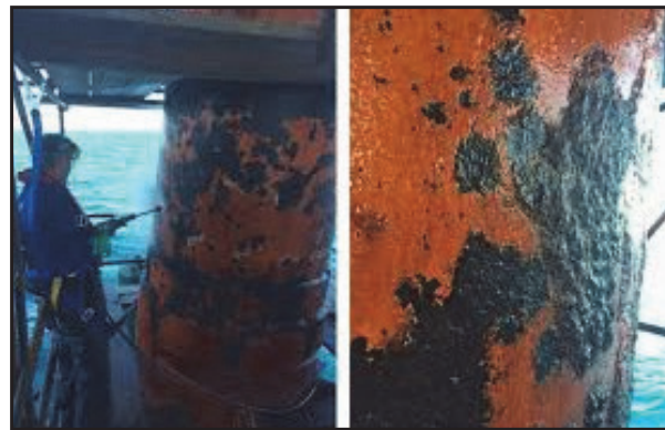
Figure 8. Corrosion formation on an underwater metal surface
